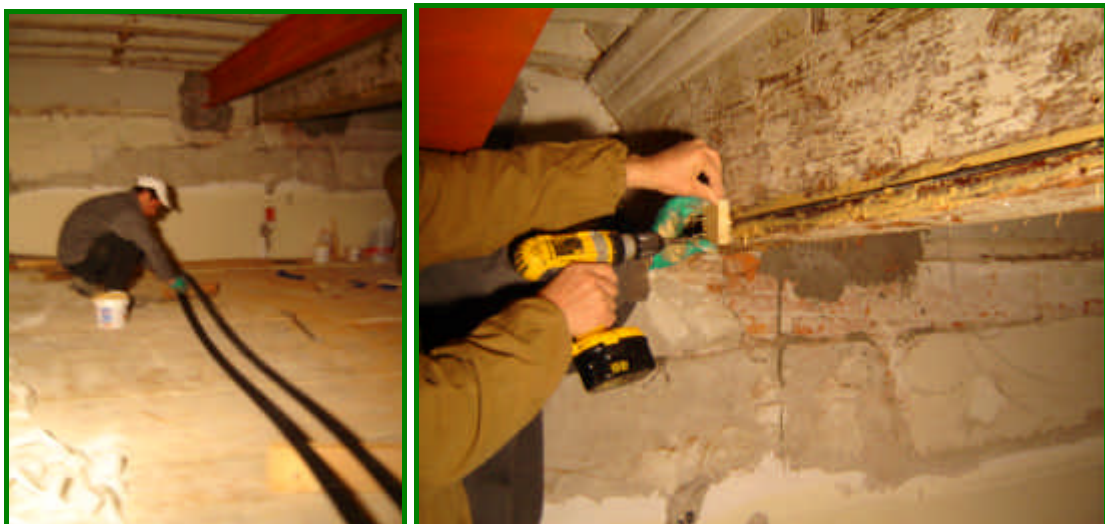
Left: peeling and applying the adhesive on the CFRP plates. Right: pushing the CFRP plates with a plywood block machined with a "T" section.
